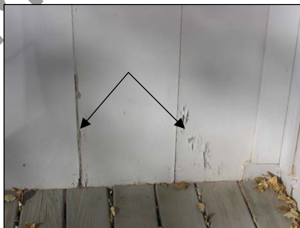
Peeling paint at the front entry.
