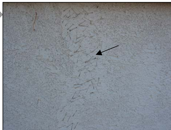
Evidence of previous repairs to surface cracking at the west wall of the addition.
